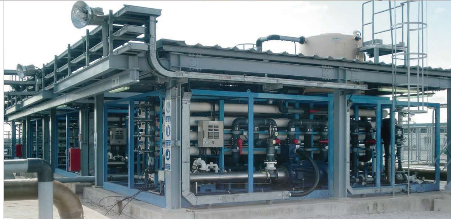
Seawater desalination plant
