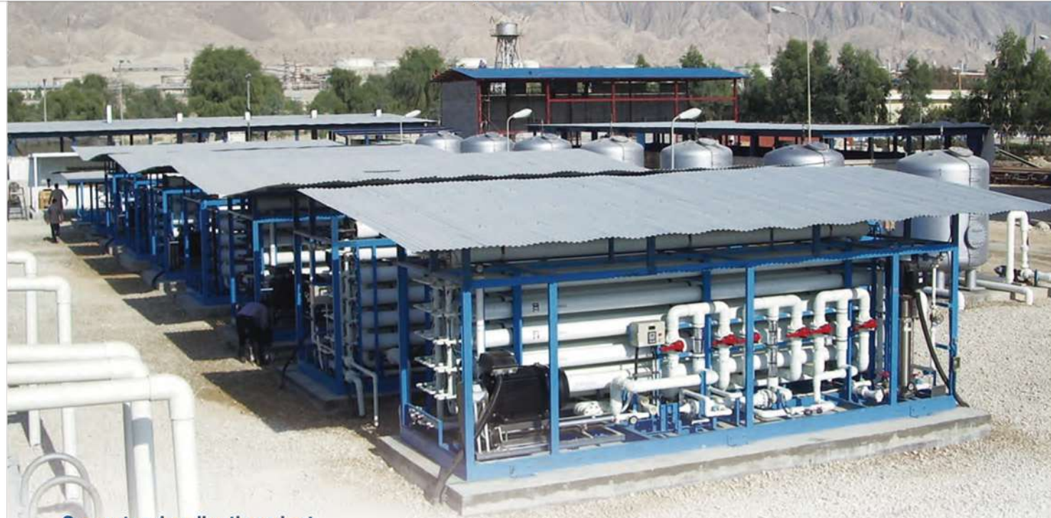
Seawater desalination plant
